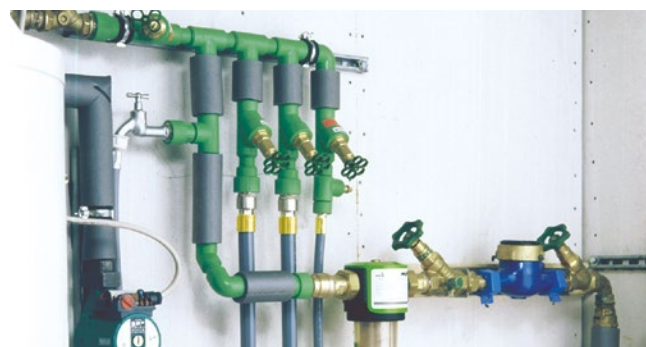
House connection station
