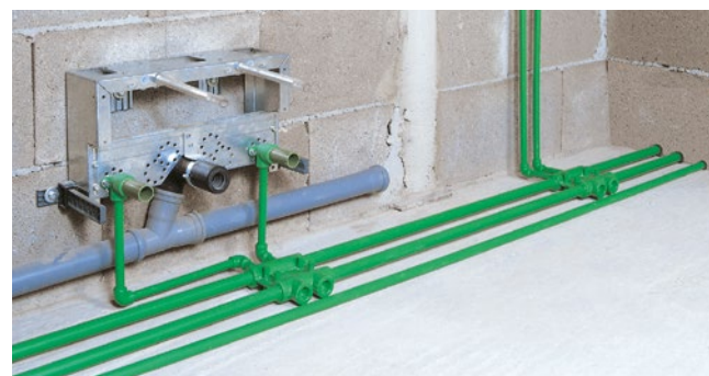
Floor distribution with distribution blocks
