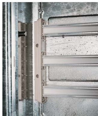
Sliding busbar counteracts damages from frost heave.
